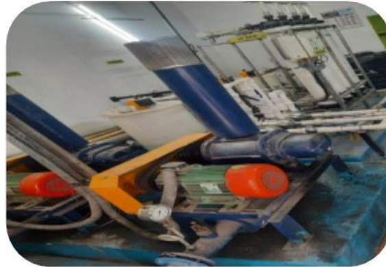
Sewage treatment plant Sewage is pretreated before its let to environment Treated water used for gardening
