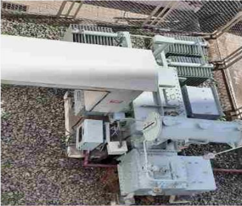
Transformer and transformer bus duct corrosion formed - cleaned and repainted
