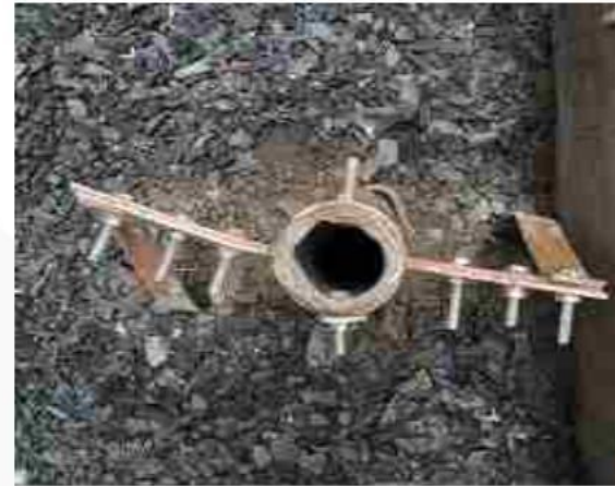
All earth pits SS bolt and nuts fixed for better earthing
